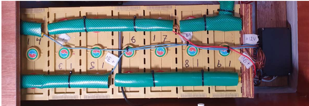
200Ah battery built from Winston LFP cells in a 2P4S configuration.
