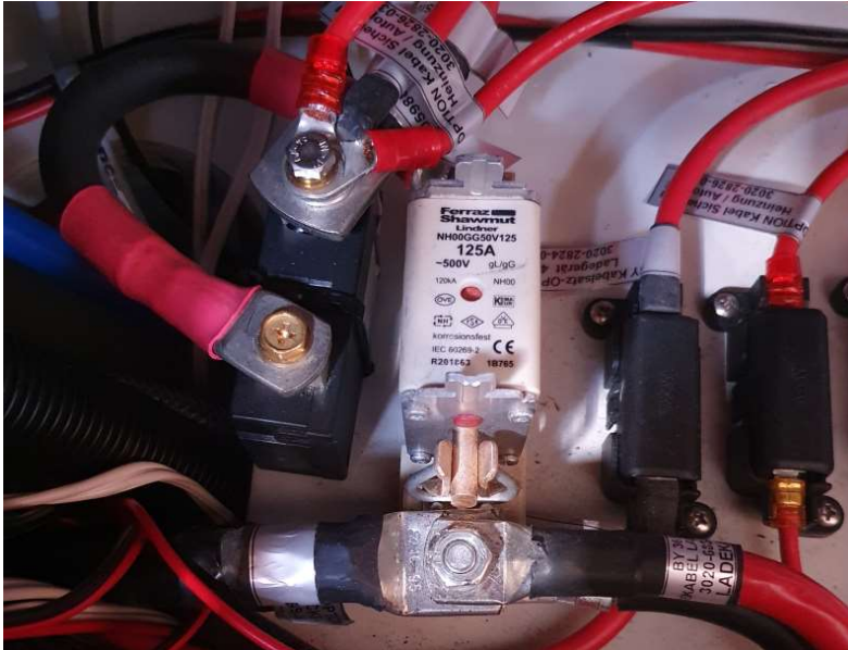
A bistable 100 A capable relay installed beside the main fuse, used to handle low voltage events.
