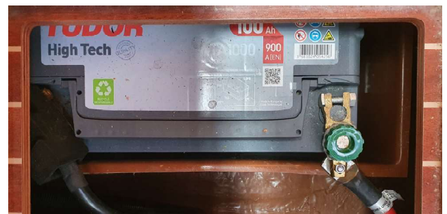
100 Ah backup battery
